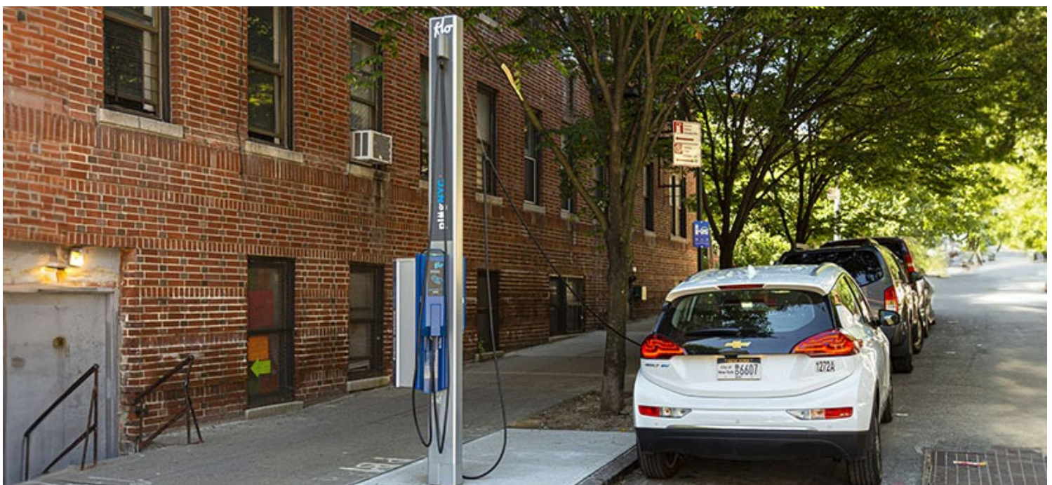
New York City curbside charging station | NYC DOT
